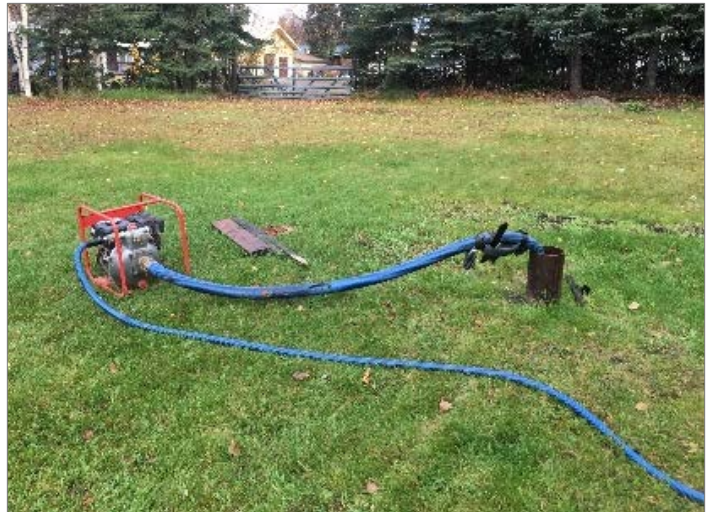
Exhibit 2-8: Photograph of Owner-Supplied Generator Pump
